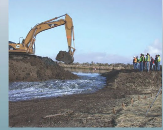
Levee breach, October 31, 2001. Photo courtesy of Chuck Morton, Caltrans.
